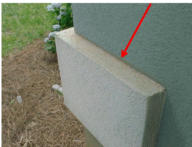
Some quoins have failing sealants - touch up all as
