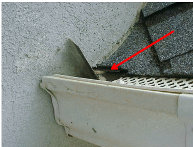
Gap in flashing overlap - high readings / poss damage below
