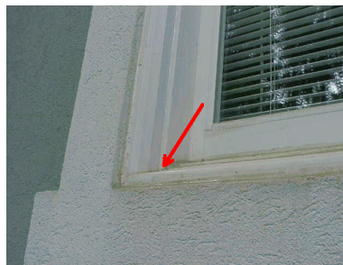
Some failed sealants noted at miters - touch up all as
