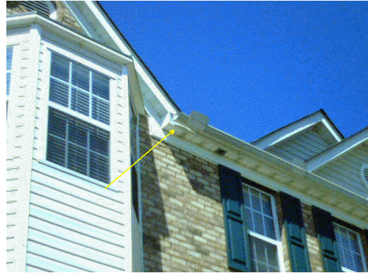
Re-attach the loose gutter at the front of the home.
